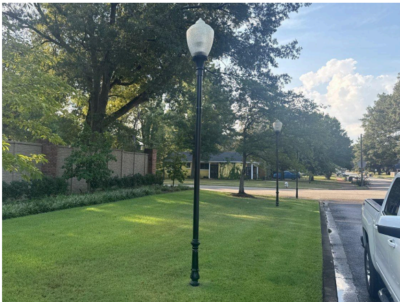
Lighting pole and fixtures
