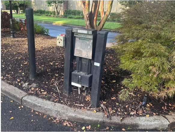
Automatic gate entry control system
