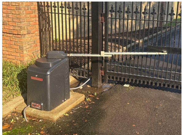
Automatic gate entry opener
